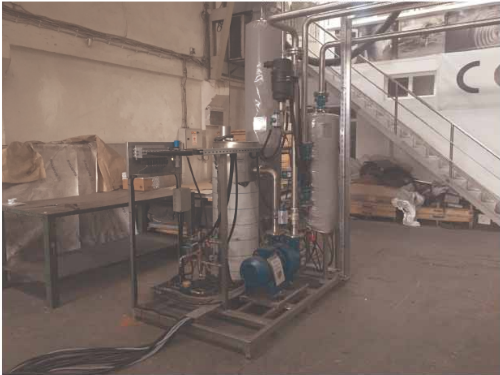
15 M3 STERILIZER MACHINE PARK VIEW – STEAM GENERATOR- ENGINES- HEATER – SCRUBBER
