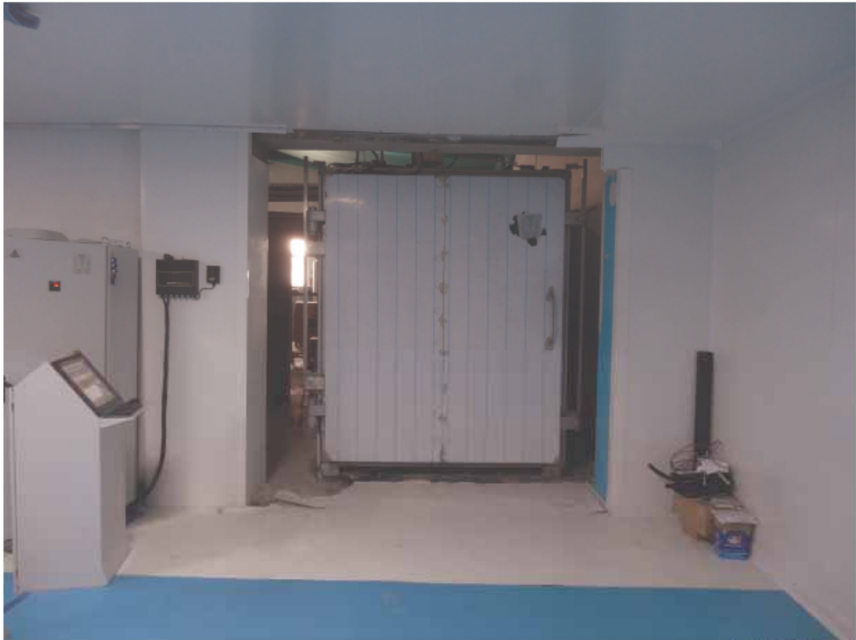
10 M3 STERILIZER * DOOR CLOSED VIEW – ETO GAS DETECTOR – KIOSK – ELECTRICAL PANEL
