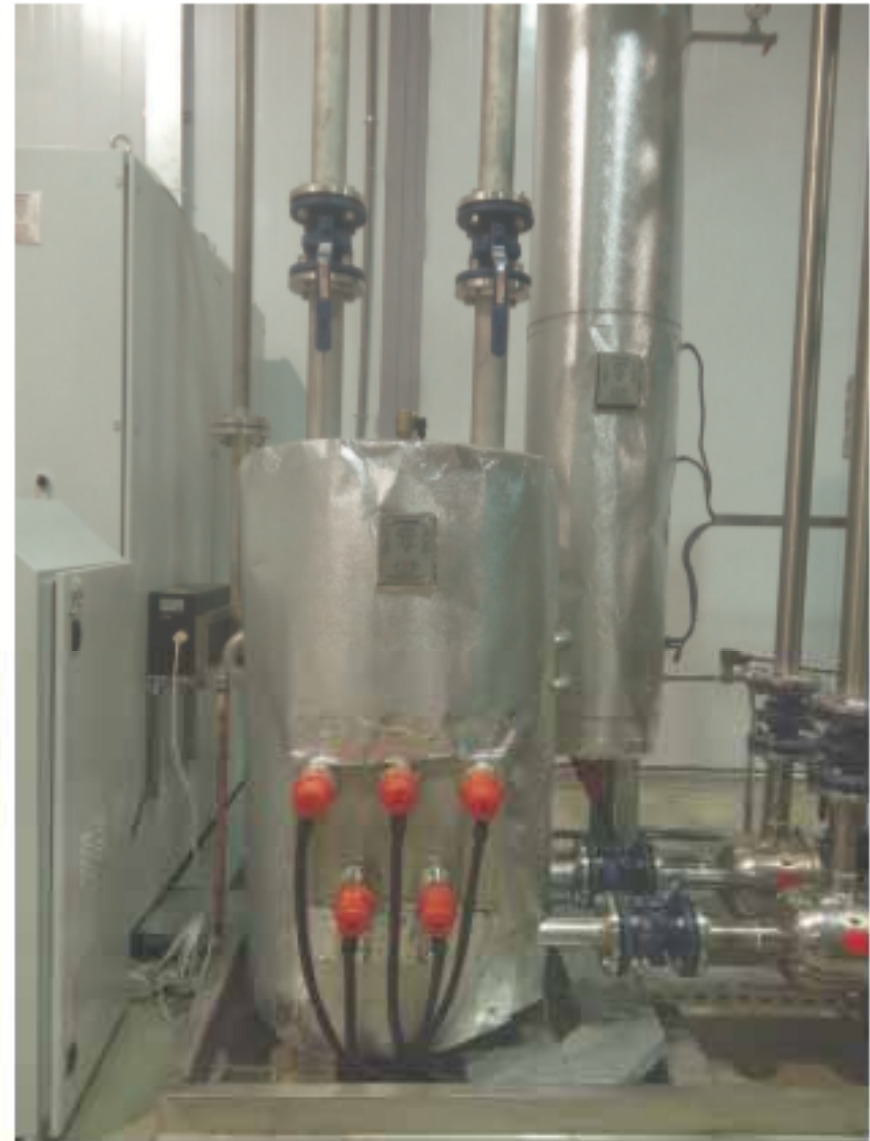
SYSTEM HEATING TANK
